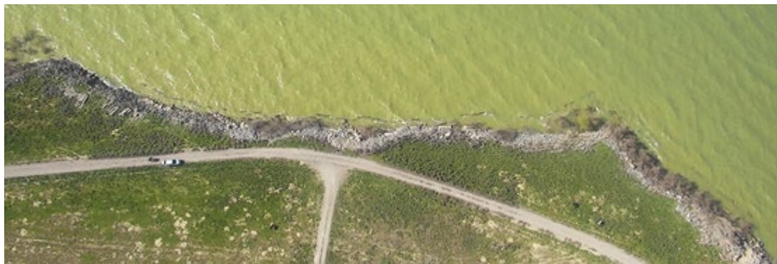
Fig.4. Erosion-prone area (drone image, 2021-04-22)
